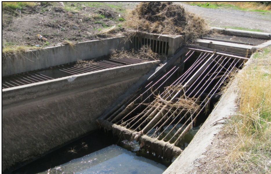
Trash rack at the entrance to an inverse siphon section.
