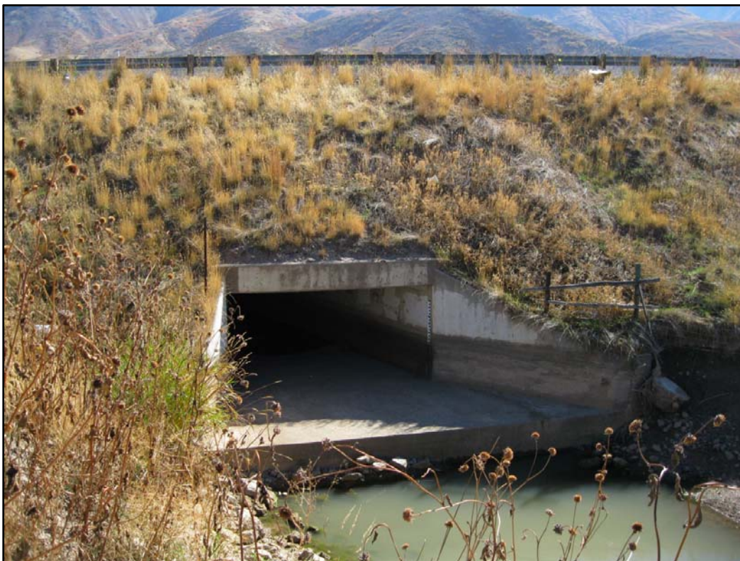
The elevation of the tunnel floor is approximately 18 inches above the downstream canal.
